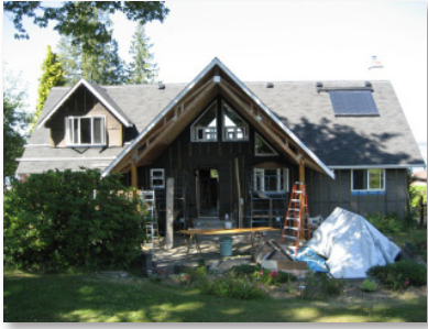
RESIDENTIAL INSTALL, SALT AIR BC Source: Via Solar
