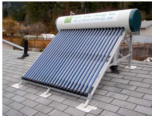
GLOBE SOLAR SYSTEM IN NELSON Source: Globe Solar
